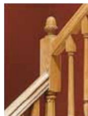
Handrail runs straight into the top block of the newel post at all landings.
